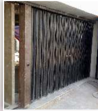
Motorised Shutter Gate
