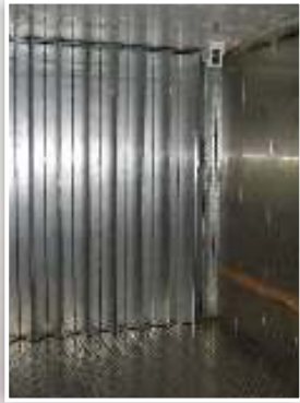
S.S. Shutter Gate
